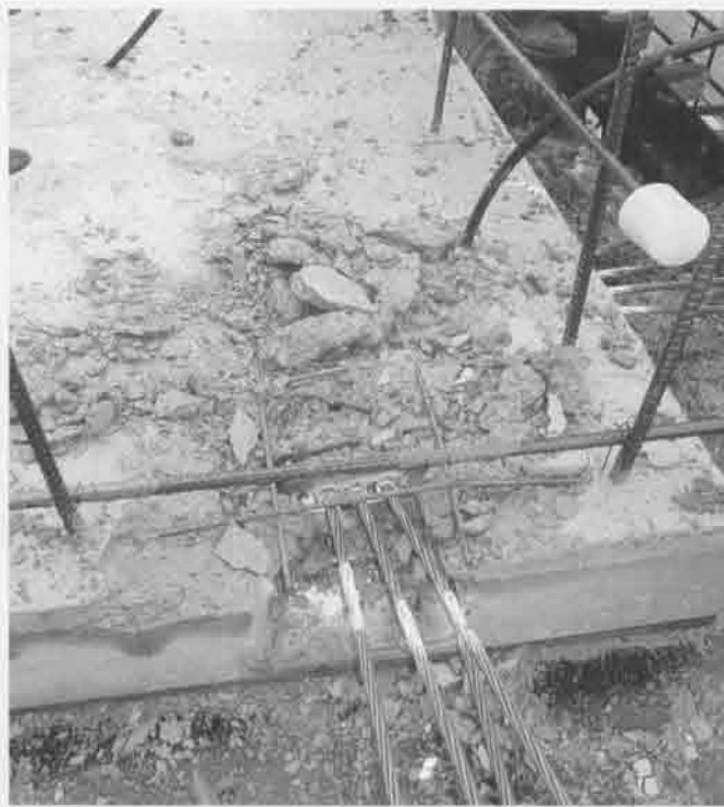
A photo of anchorage failure in cold weather.
